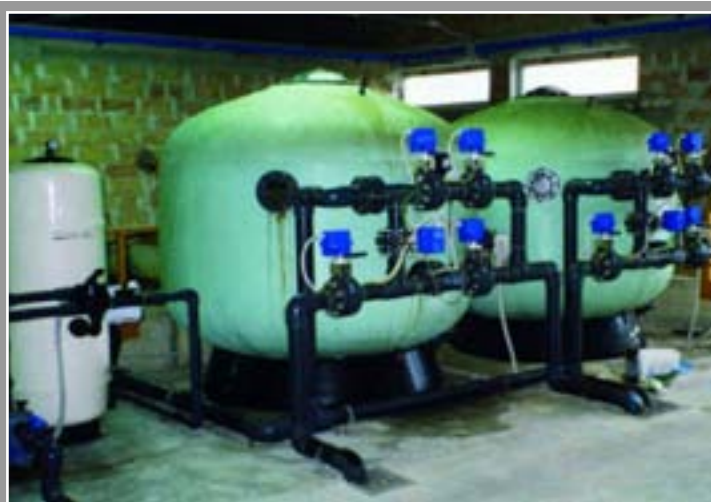
Fig. 61 - Pressurized sand filter
