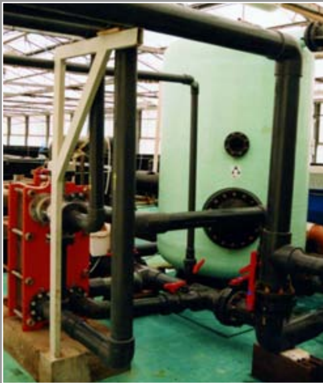
Fig. 65 - Pressure biofilter and plate heat exchanger
